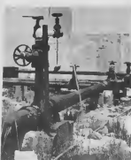
Water left running like this the water and money wasted. Report laaka — they are apanalva.
